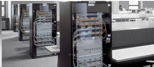
Individual Cool-Rack cabinets
